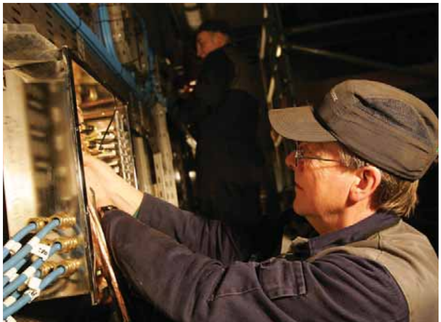
Hands on: a Mech-Tool worker installs an electric panel on a compressor skid unit
