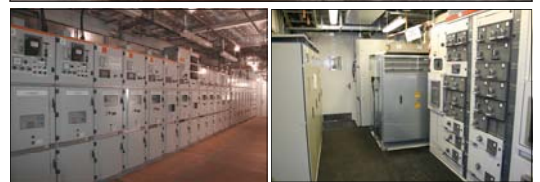
Fire & Blast Rated Switchgear Module
